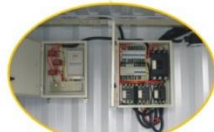
■ 电表、开关柜 Electricity meter, power cabinet
